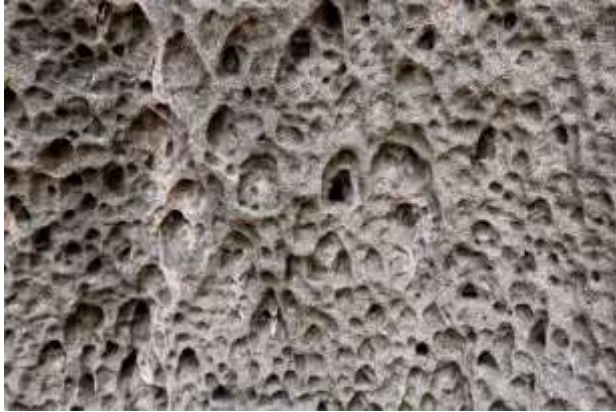
damaged rock because of water
